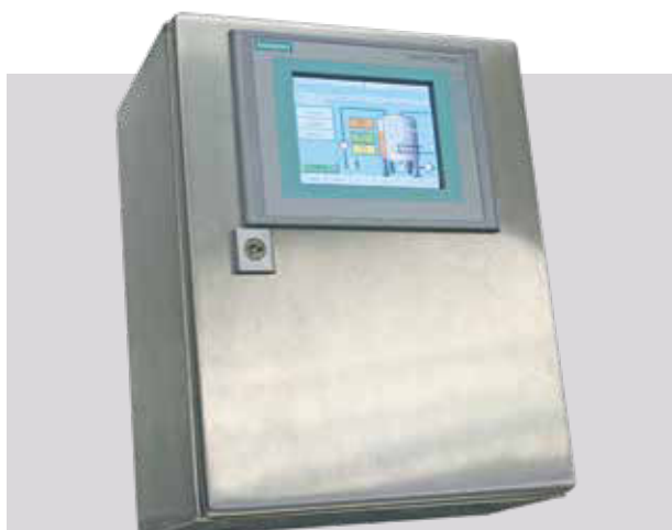
Transmitter S7 Control Cabinet with Touch Panel
